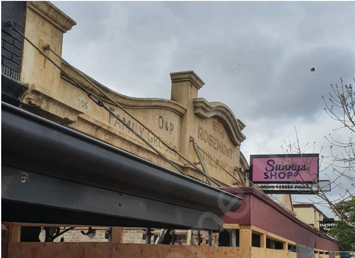
Photo 1 – View of wall rotation over the western Prospect Road footpath
