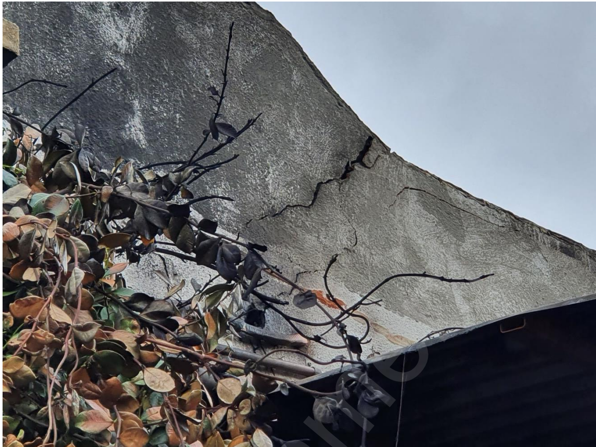
Photo 5 – Cracking to eastern end of northern elevation
