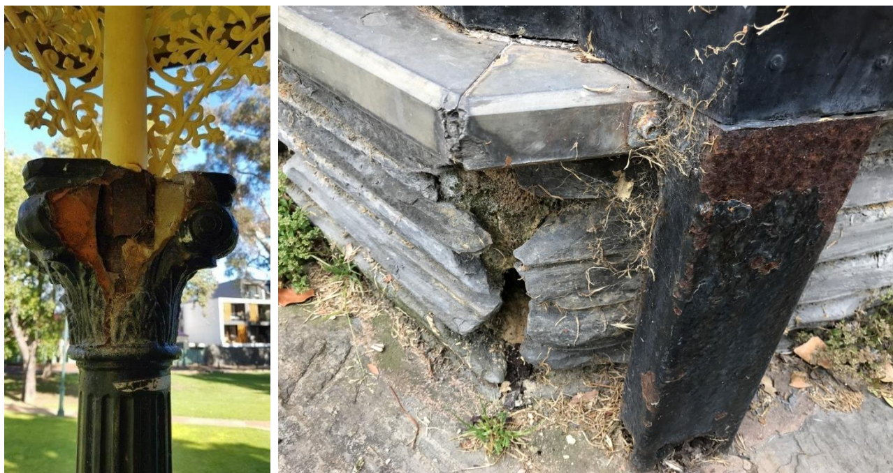
Figure 1: St Helens Rotunda Structural Defects
